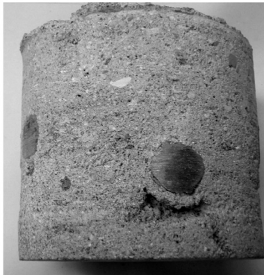
Dry-mix shotcrete, intersection #4 bars, mid size void too large to be a Core Grade #2.
